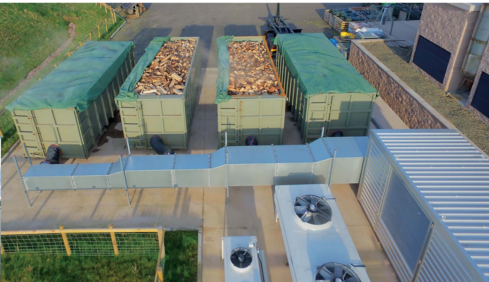
Biogas plant in England with a L-ENZ 370, air duct and four drying containers.
