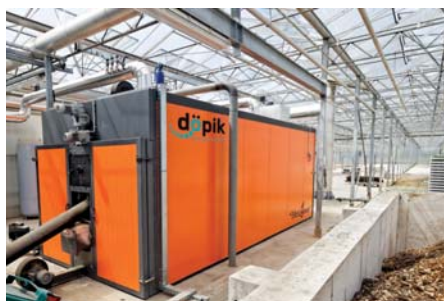
Woodchip boiler with storage bunker.
